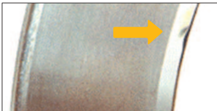
Dings and dents in the bearing surfaces indicates a drift was used during installation.
