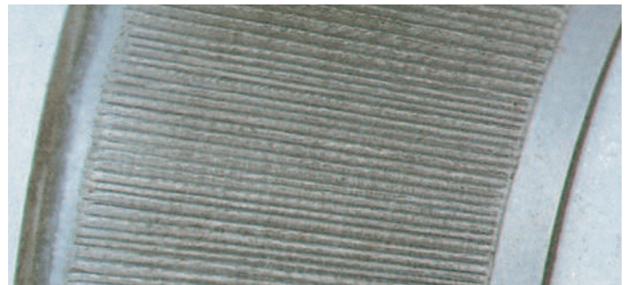
Light pitting can be caused by electrical arcing. The probable cause is electrical welding grounded through the shaft.
